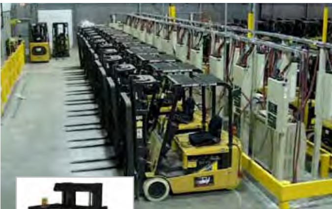
Charging station for battery operated forklifts
