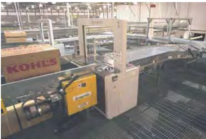
A sorter conveyor with scanner.
